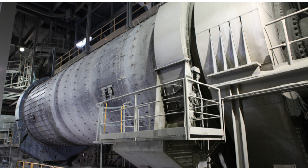
Cement mill. Alcalá de Guadaíra factory, in Seville (Spain).
